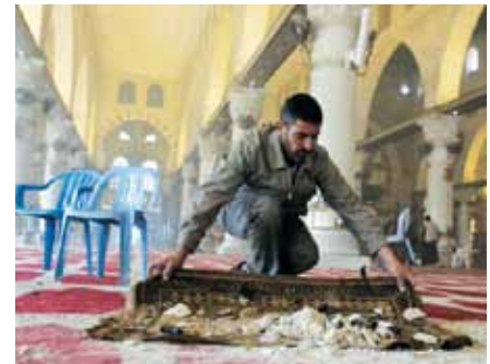
Damages inside Al-Aqsa Mosque after the Israeli 5 Nov. 2014 assault
